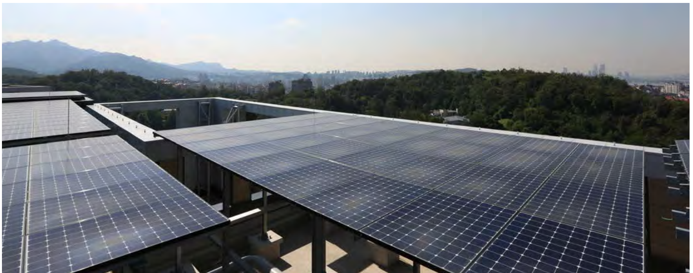
Majestar City Tower, an Invesco property located in Asia that produces solar energy on-site and is consumed on-site by the landlord.
